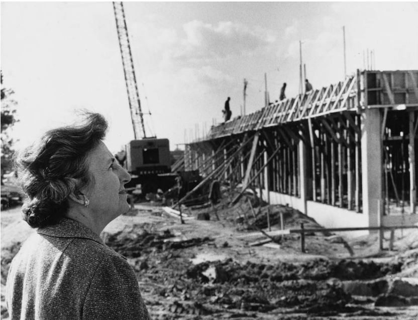
Cone looks on as the J. Murrey Atkins Library building is constructed, circa 1960–61.
